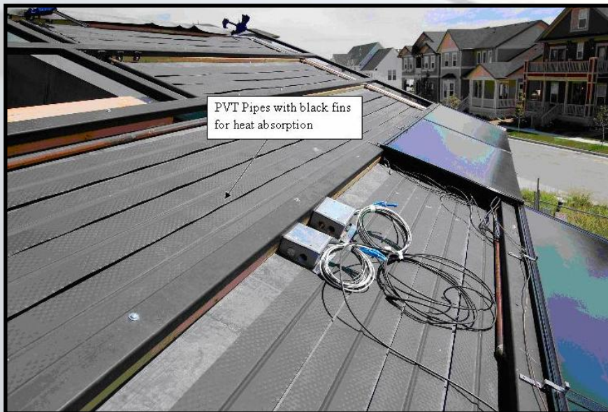
Figure 1: PVT system with pipes and fins on the University of Colorado 2007 Solar Decathlon house.
